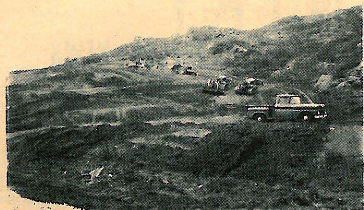
The freeway continues to move toward Alpine, as shown by the new construction on the route.
